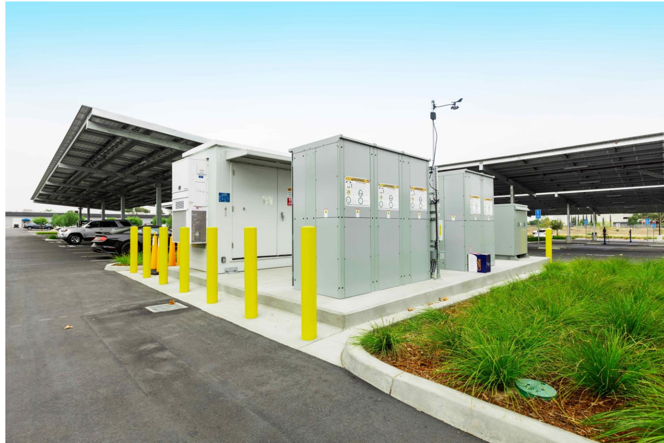
Battery energy storage system and solar PV (Source: PowerFlex)
