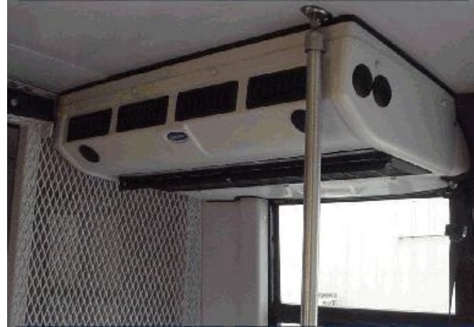
Bus air conditioner (Source: Nesco)
