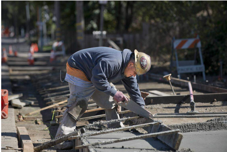
A construction worker cuts lumber while building a sidewalk along Marconi Avenue in Carmichael in 2013. Sidewalk construction projects like this are often built in phases as local agencies compete for limited state Active Transportation Program grants to fund pedestrian safety improvements. Hector Amezcua hamezcua@sacbee.com
