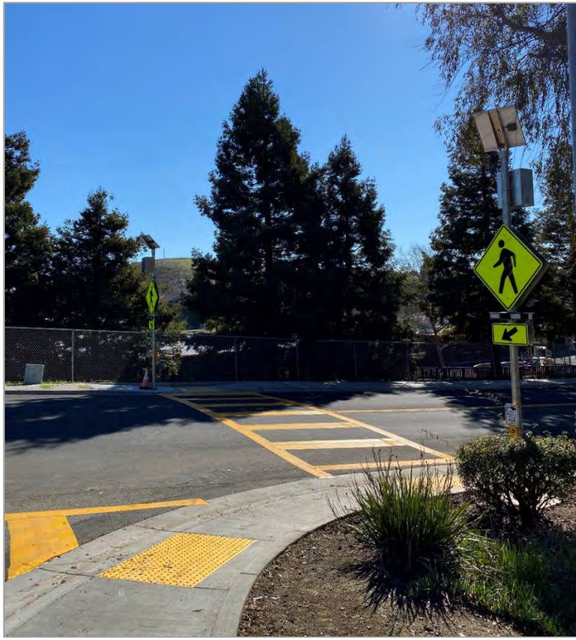
Joe Henderson Elementary, Benicia Rapid Rectangular Flashing Beacon (RRFB)
